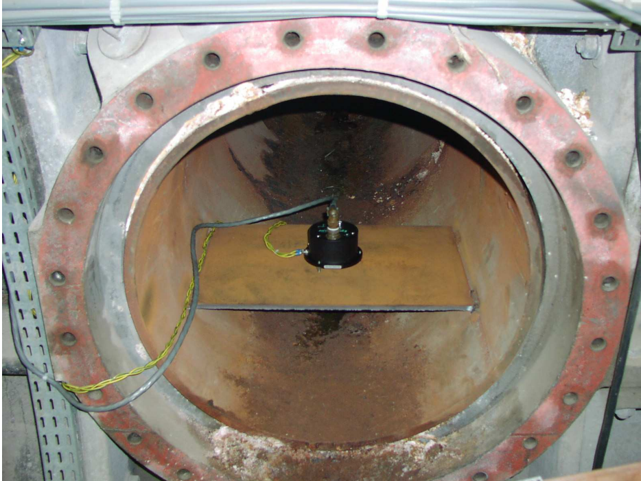
Figure 5. Triaxial EpiSensor accelerometer in the tunnel, connected to the K2 using a 305 m long cable.
