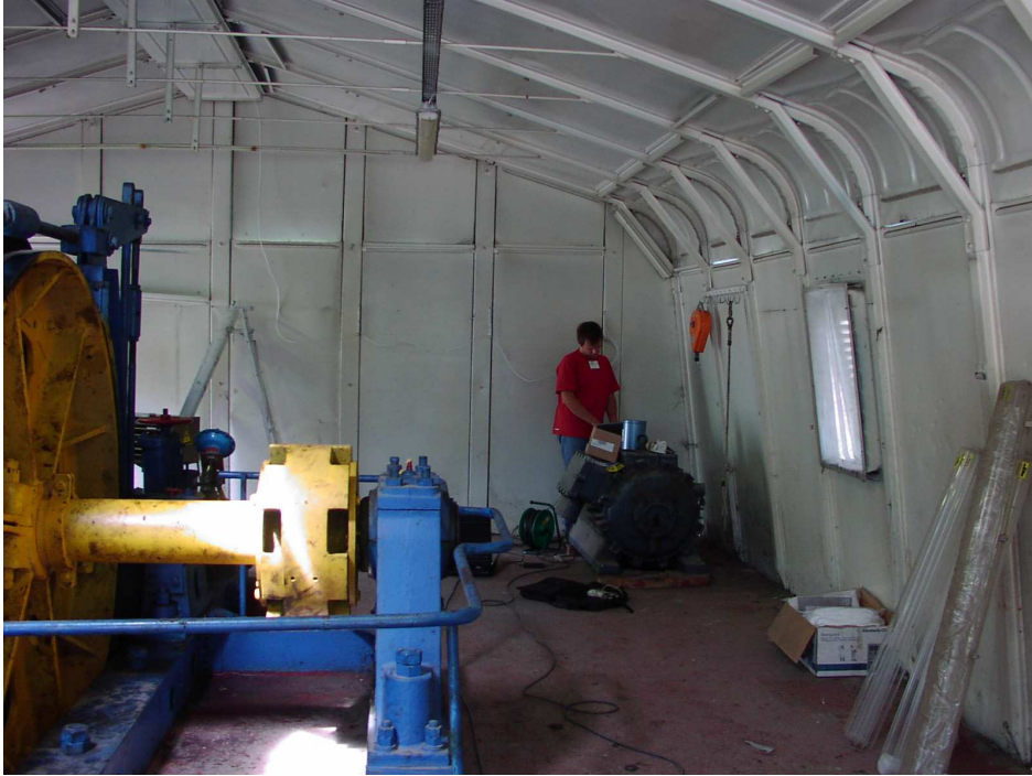
Figure 3. Installing the K2 accelerograph in the shelter housing the old lift machinery.
